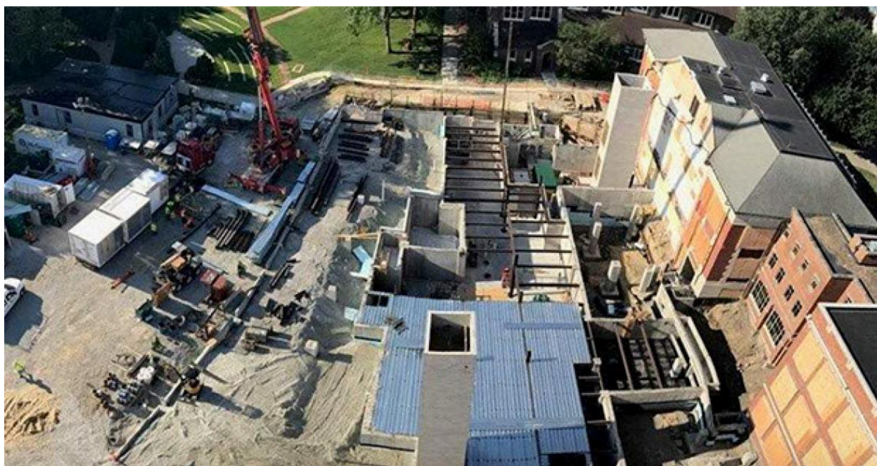
Construction of the HSSC, Carnegie pictured on the right, 2017. Publisher: Grinnell College
